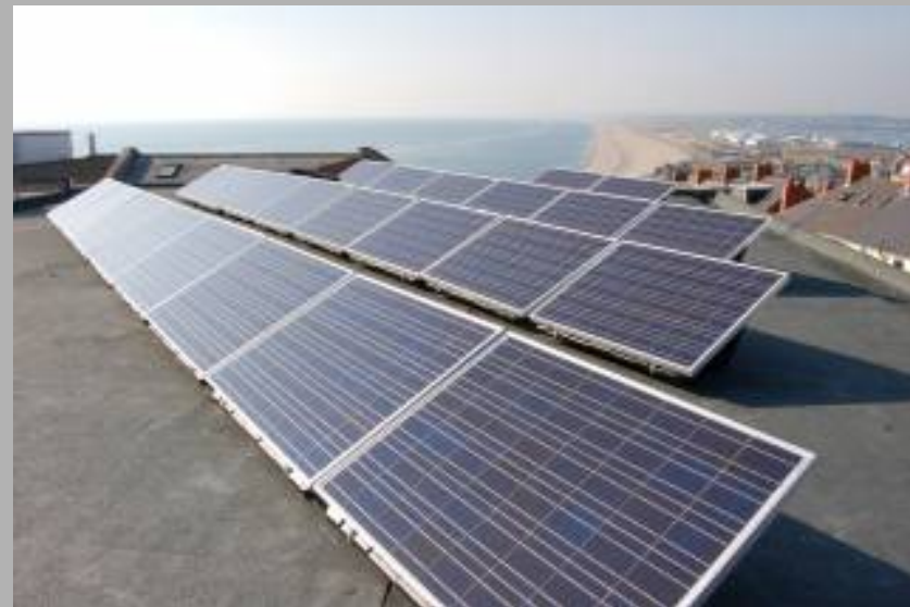
Solar PV at Underhill School, Portland
